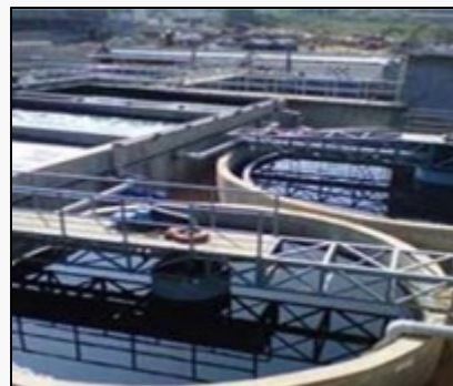
Common Effluent Treatment
